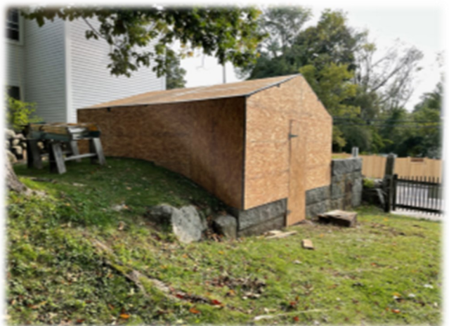
The completed enclosure. As of Oct. 1, the mason has removed and replaced the old brick facing
