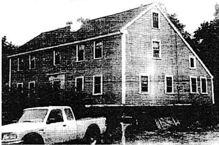
The Historic Holt house is being restored, original bricks will be washed and used again.
